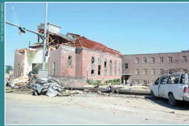
Alberta Baptist Church, above, and the surrounding area were heavily damaged by the storm. The church has since rebuilt, and construction continues in the region.
